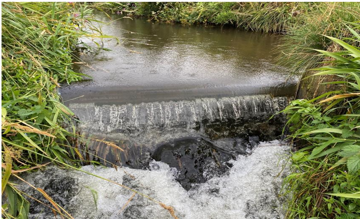
Fig 3. Below showing boards placed at the top of the Ebrie burn channel causing obstruction.
