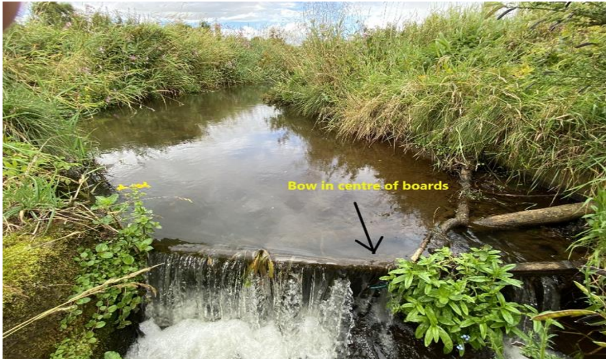
Fig 2, above showing bow in centre of boards at top of abstraction channel
